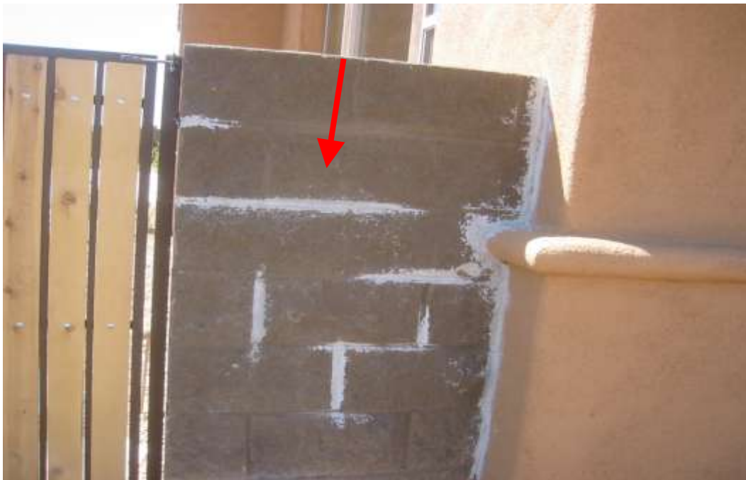
Touch-up painting needed on back yard block fence/wall.
