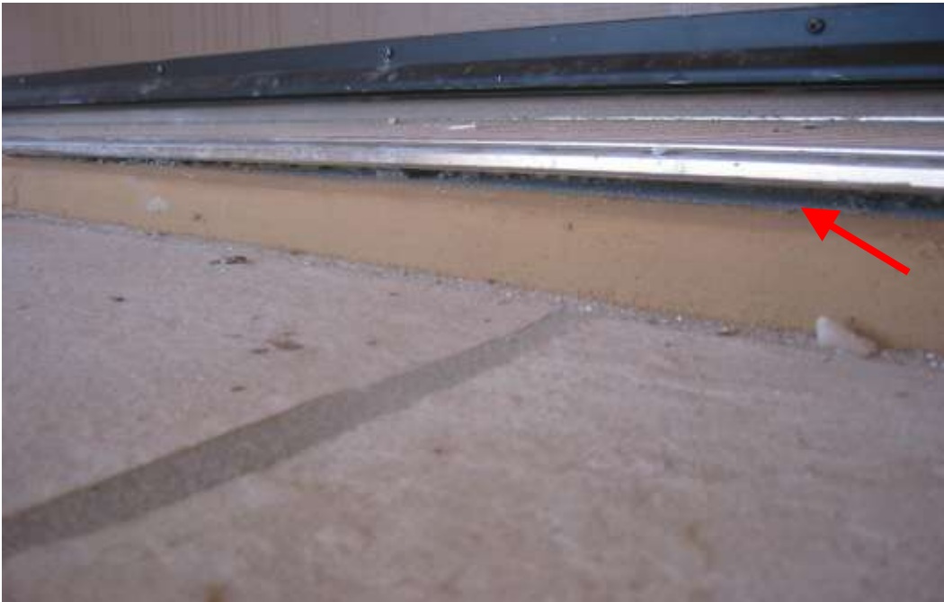
Gaps below door thresholds.
