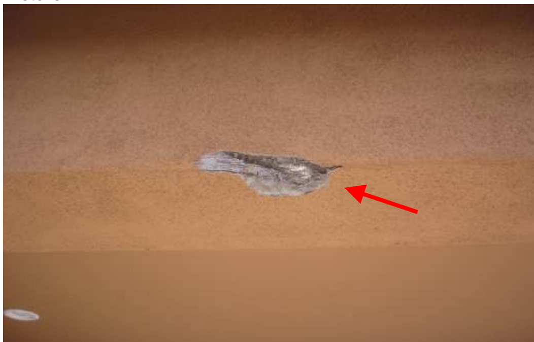
Stucco damage on lower corner of carport/breezeway.
