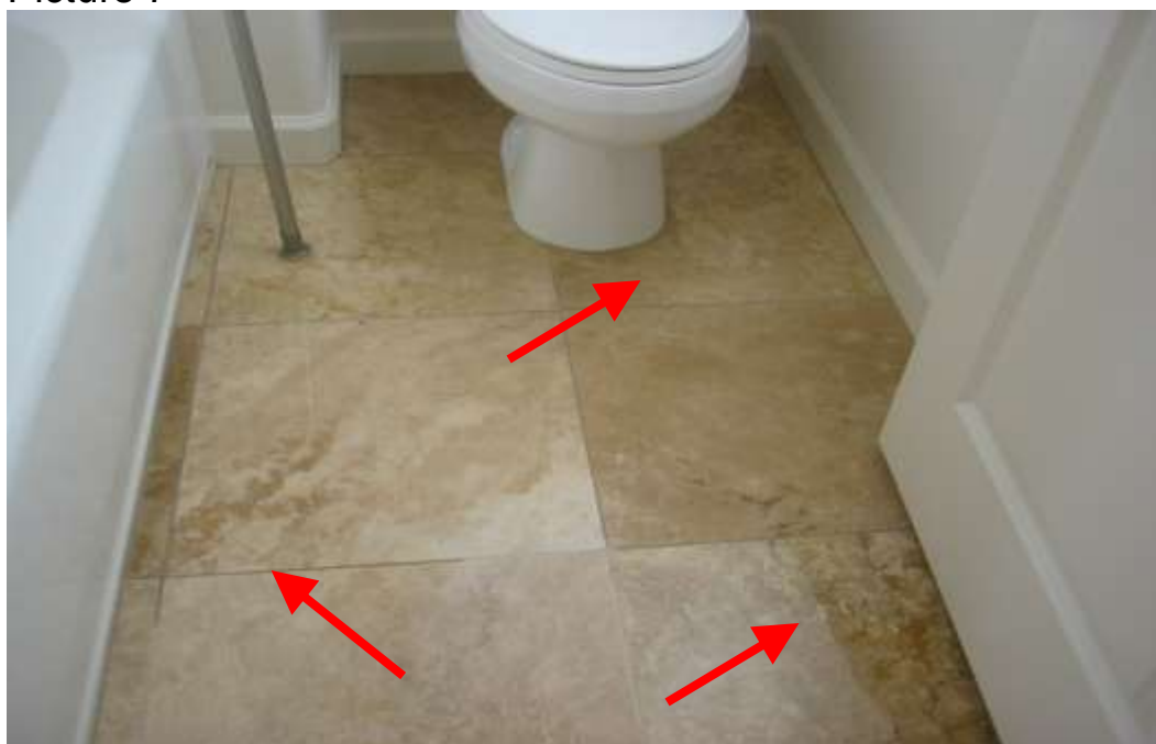
Water on hallway bathroom floor from bath tub (drain leak below tub?).
