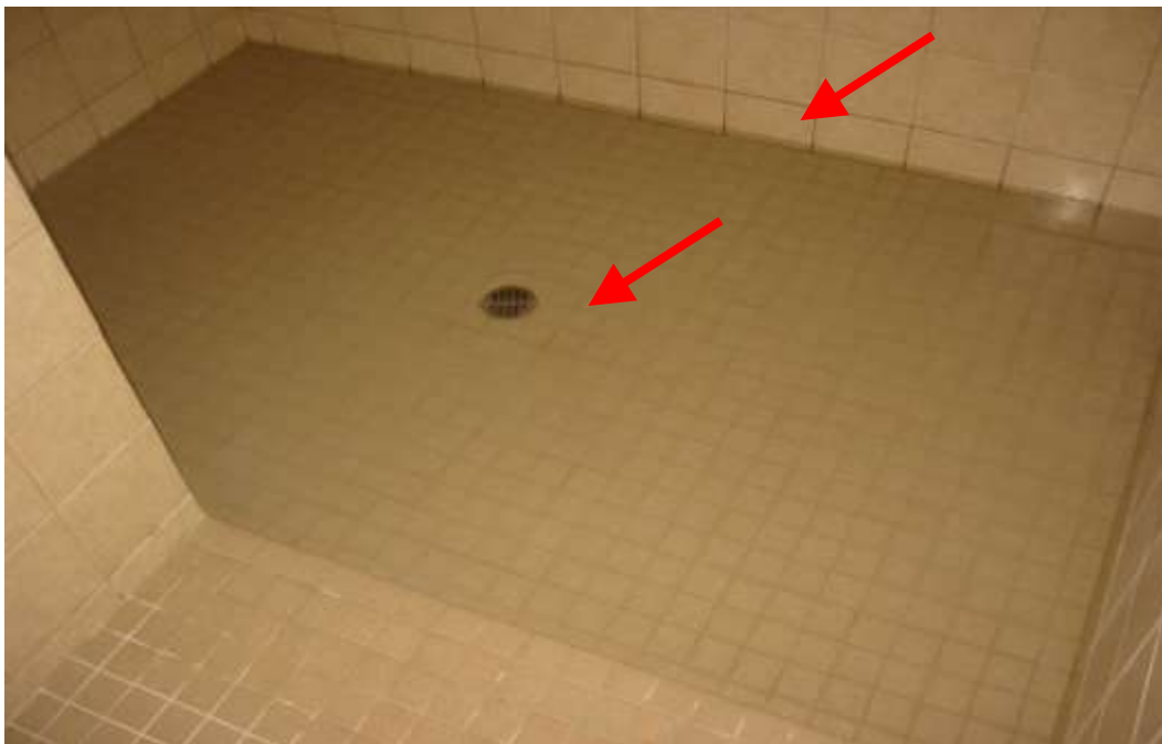
Water in master bathroom shower stall from bath tub draining.
