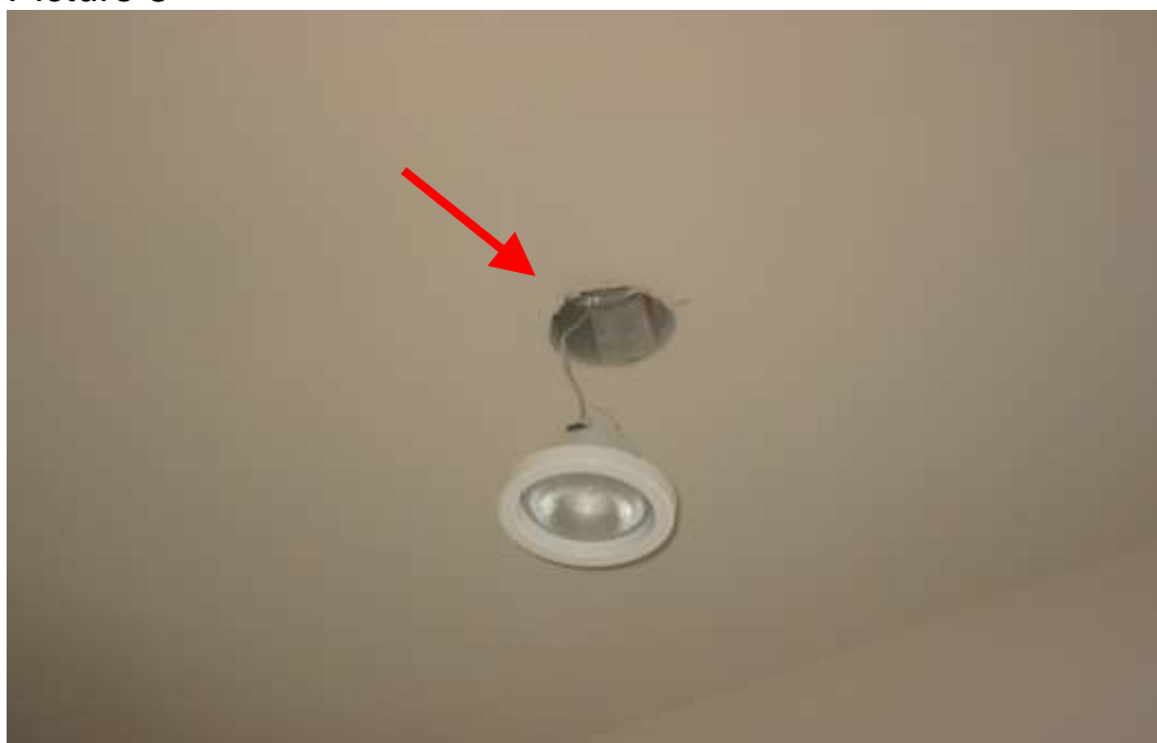
Light in master bathroom shower stall loose.
